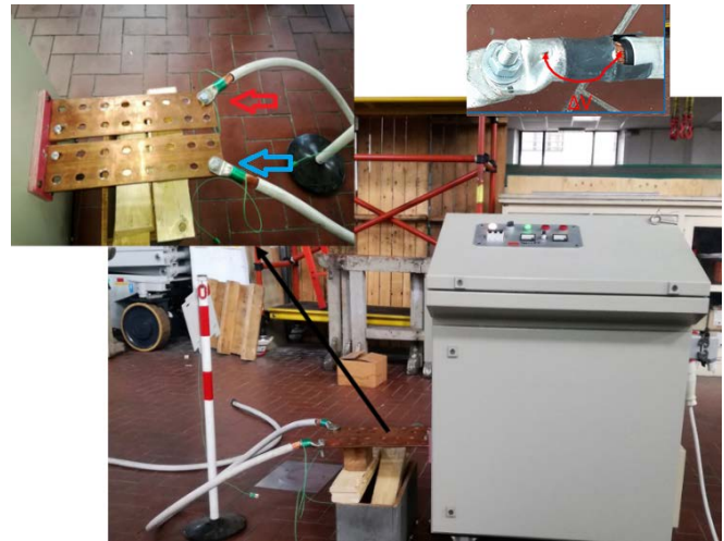
Fig.3. Measurement setup with zoom of the connection between the cable lugs and the bars and of the place where voltage measurements have been made.
