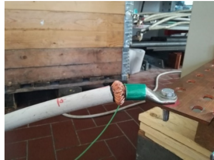
Fig.14. Swelling of the bare cable area.
