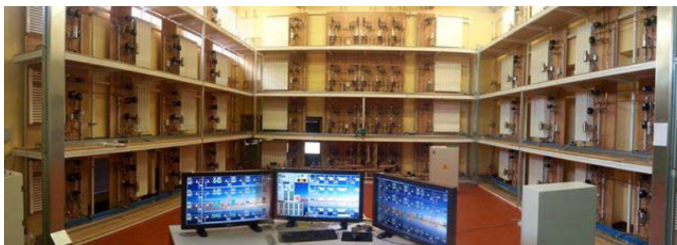
Fig. 1. Overview of the thermo-hydraulic circuit of the INRIM central heating system simulator.
