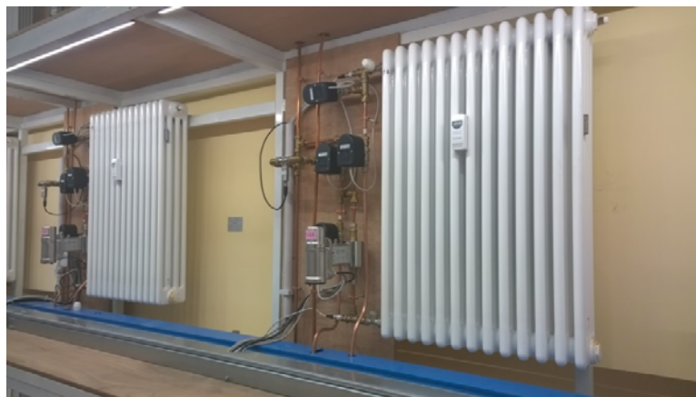
Fig. 12. HCAs installed at the INRIM thermo-hydraulic simulator.
