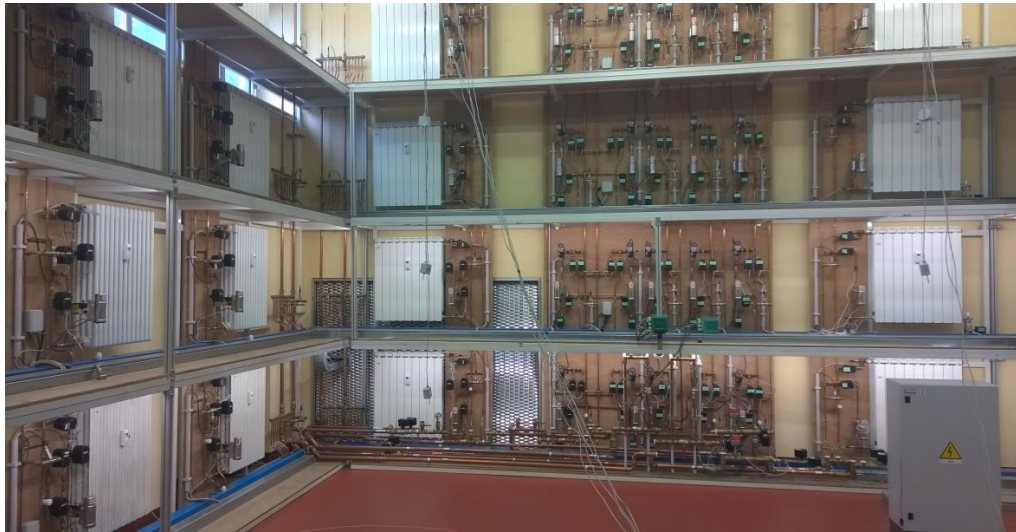
Figure 6. Experimental setup at the INRIM central heating system test facility.
